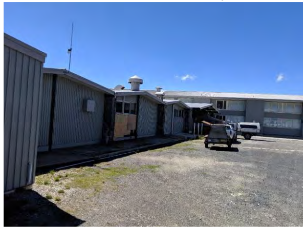
Figure 6: Photo of the southern side of the hotel and location of the single storey addition comprising of the garbage and store room
