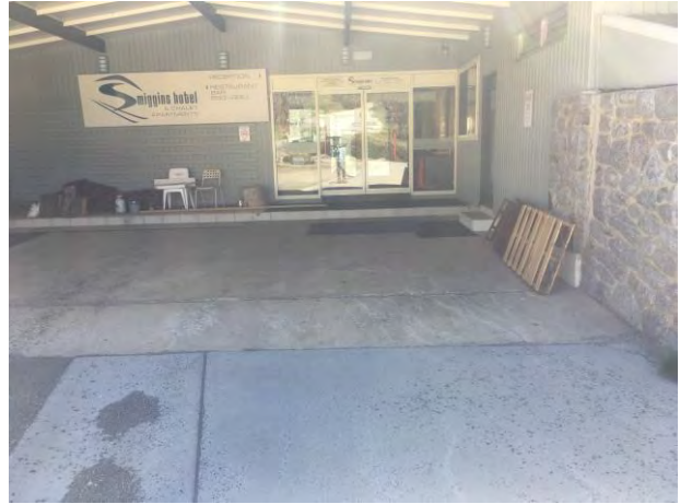
Figure 4: Photo of southern side of the hotel and location of the access ramp
